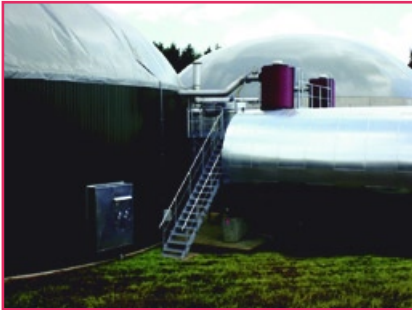
Biogas Anlage Photo: Archea Biogas N.V
